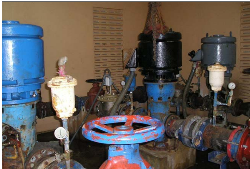
Figure 13-4 – Interior View of Brigade Booster Pump Station
