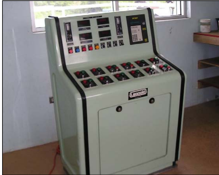
Figure 13-5 – Unused Control Console at Ugum WTP
