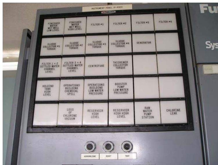
Figure 13-7 – Annunciator Panel at Ugum WTP
