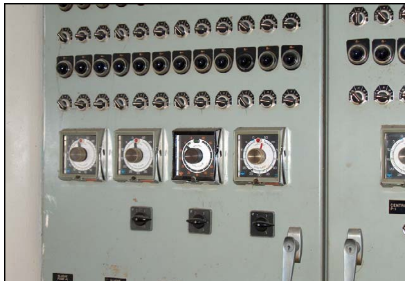
Figure 13-6 - Unused Control Panel at Hagatna STP
