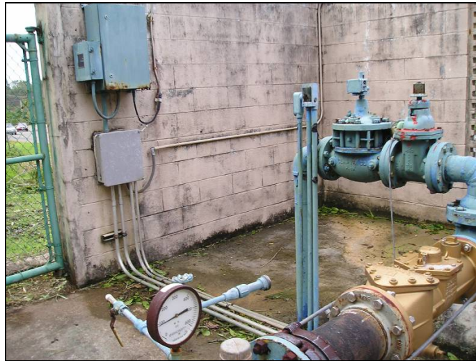
Figure 13-3 – Non-Functioning Bypass Valve and SCADA Cabinet at Station A-03
