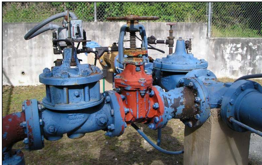
Figure 13-2 – Operational Bypass Valve at Station Y-21A
